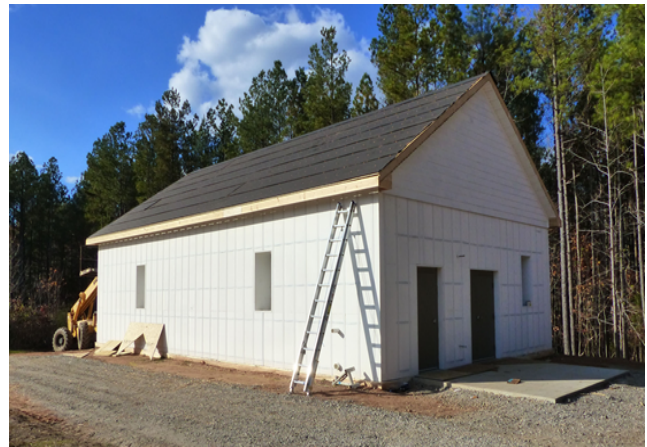
Figure 2: This is an image of the recent construction of the Energy Research Lab.
